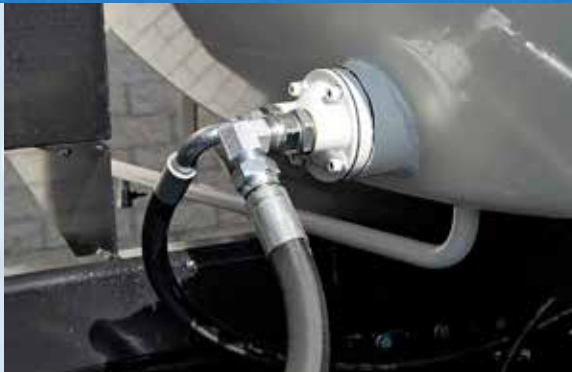
Water Inlet & Outlet
